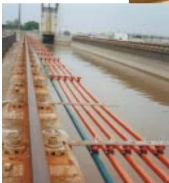
Water Treatment Works
