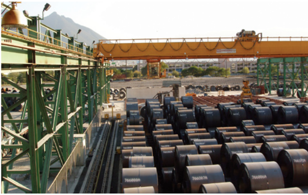
APM Steel Mill - Mexico Hevi-Bar II - 500 Amp
