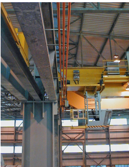
Antamina Copper Mine - Peru Hevi-Bar II - 1500 Amp
